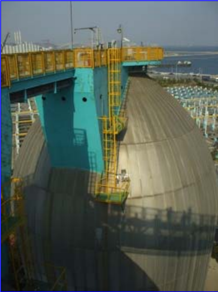
Biodigester in Ulsan, generating 4x more methane by combining solid waste and slurry
