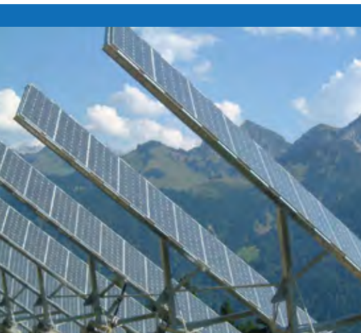
Photovoltaics at Blonz (© Gr. Walsertal BR)
